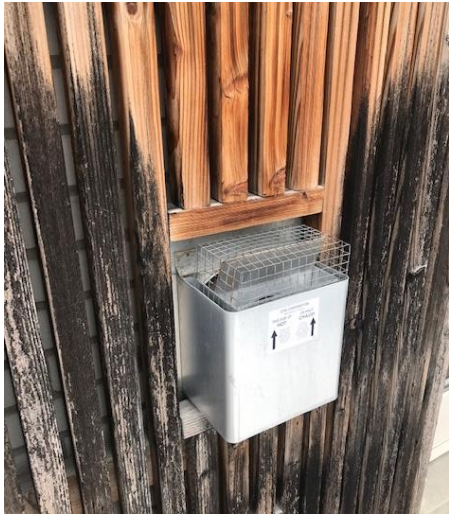
G: the direct-vent fireplace in the rear family room discharges the exhaust gases around wood siding. A metal barrier is required at the top of the exhaust vent.
